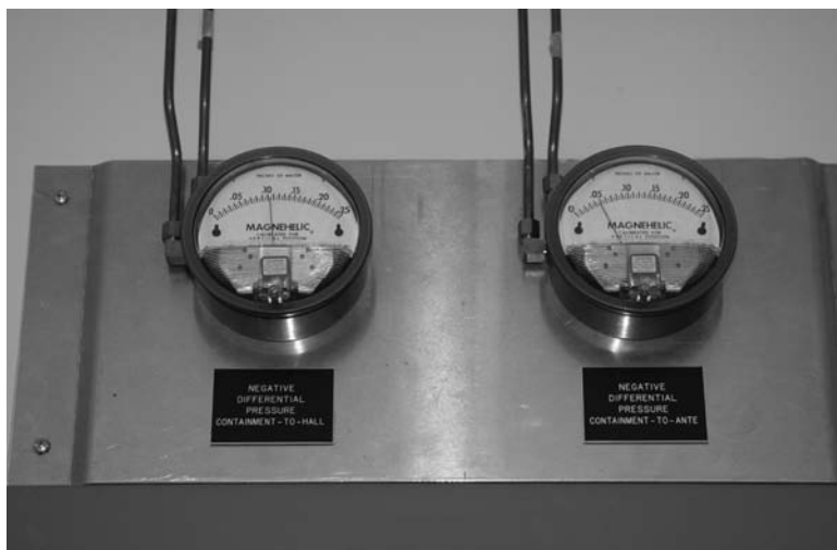
Figure 17.2 Magnahelic gages measuring pressure differentials between rooms in a containment facility.
